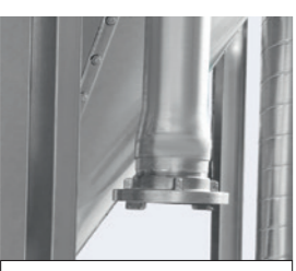
feed truck connection
